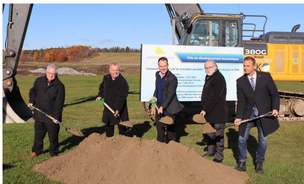
Groundbreaking at the Gatineau-Ottawa Executive Airport for a new taxiway thanks to a $3,889,845 investment by the Government of Canada
